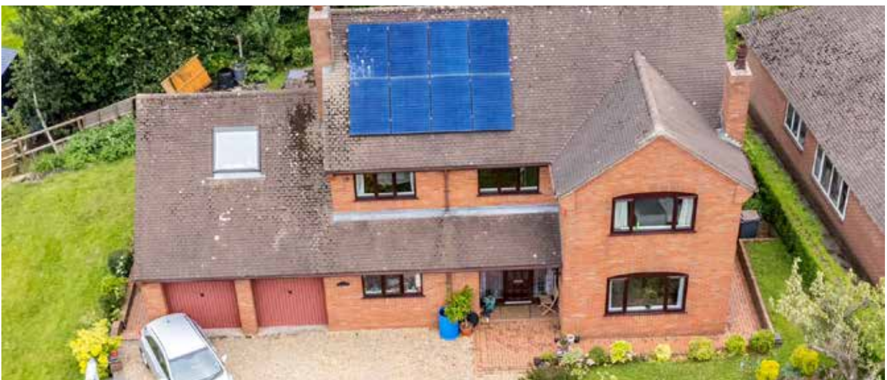
Figure 7.5, Example of local solar panels used for local energy generation
